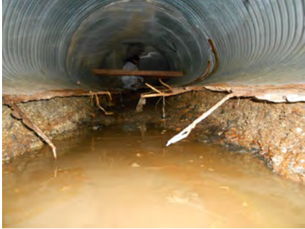
Invert needed to be repaired prior to application of geopolymer
