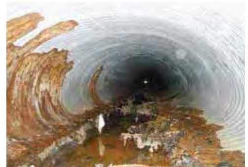
Severely corroded CMP invert
