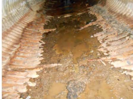
Severe invert corrosion
